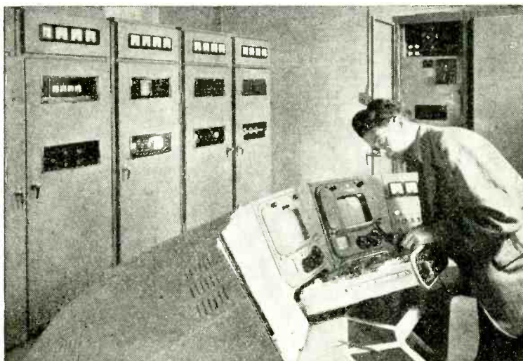
HOLME MOSS. Medium-power stand-by transmitters (5kW vision, 2kW sound) installed by Marconi's at the B.B.C.'s northern television station which is to be opened by the P.M.G. on October 12th. The transmitters are similar to those originally ordered for the five secondary stations.
